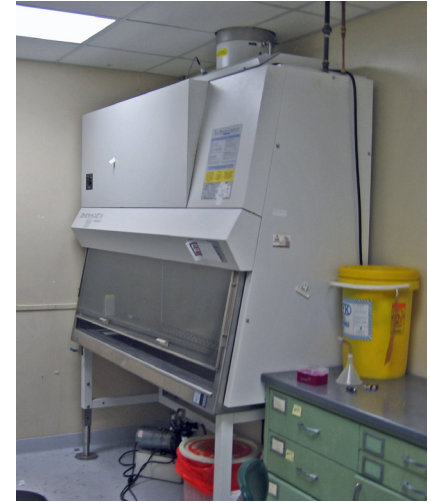
Figure 4.9: View of Level 2 Biological Safety Cabinet in Rooms 516A, 516B, 516E, and 516F.
