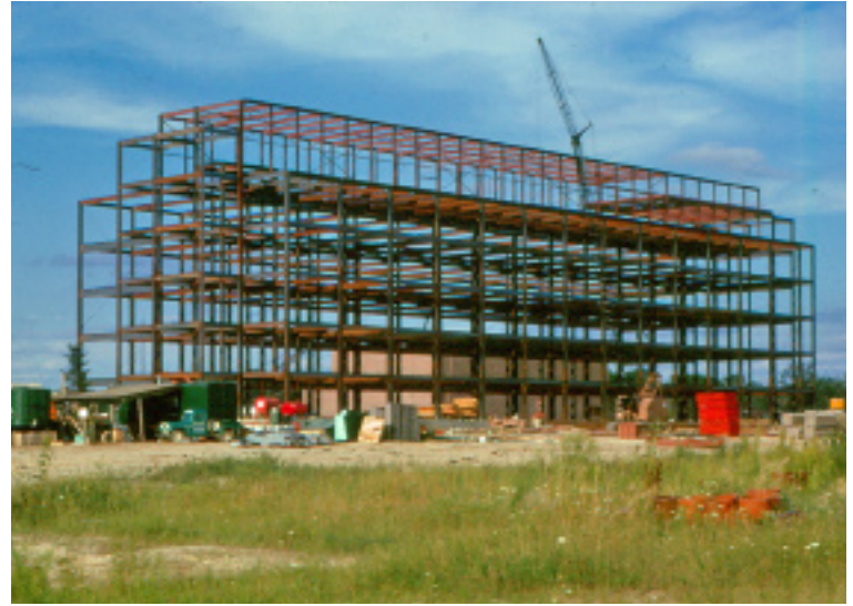
Figure 3.1: A view of the Biochemistry Building under construction in the summer of 1963. The Cyclotron Building can be seen behind the steel structure. Courtesy of Theodore Jackanicz, Ph.D. 1965. UA 16.18, Michigan State University Archives and Historical Collections, East Lansing, MI.
